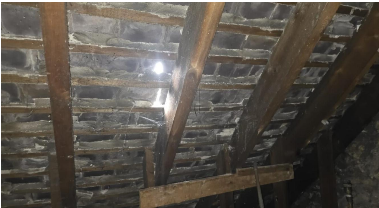
Plate 8: Image of the gaps in the internal tiles in B1 .
