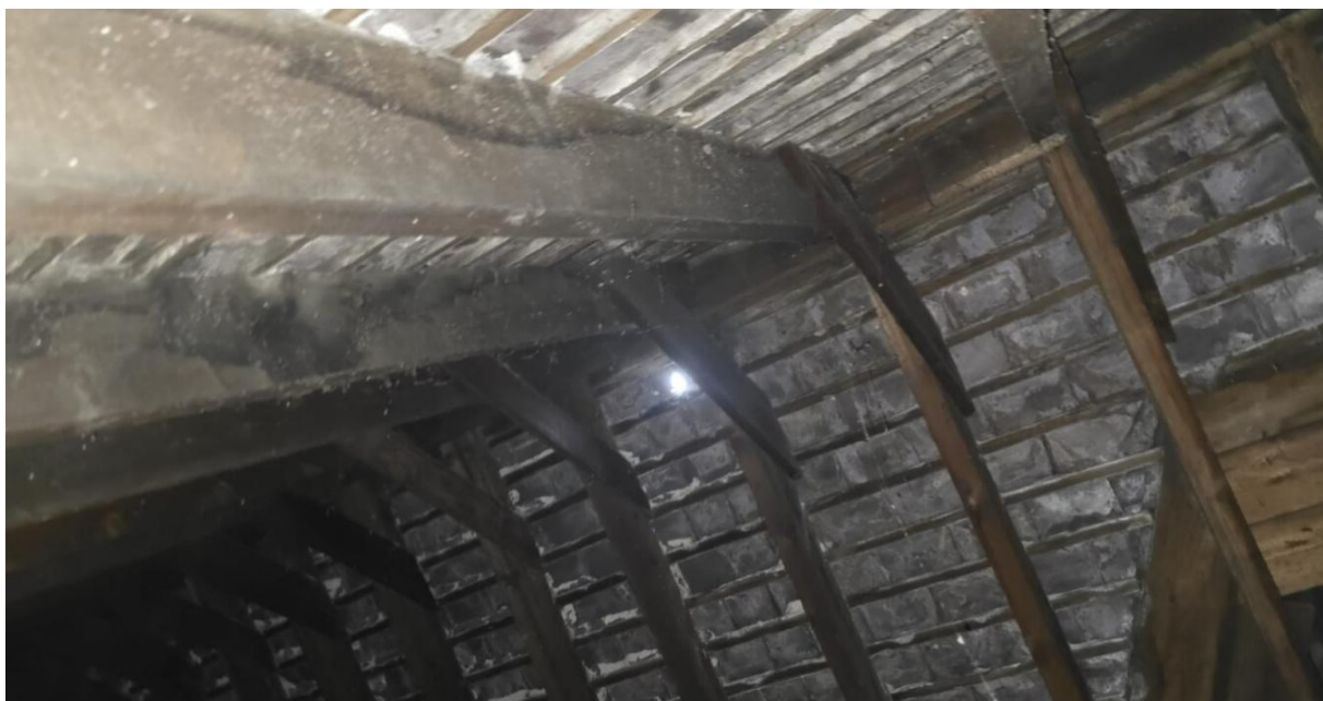
Plate 6: Image showing the gaps in the internal roof of B1 .
